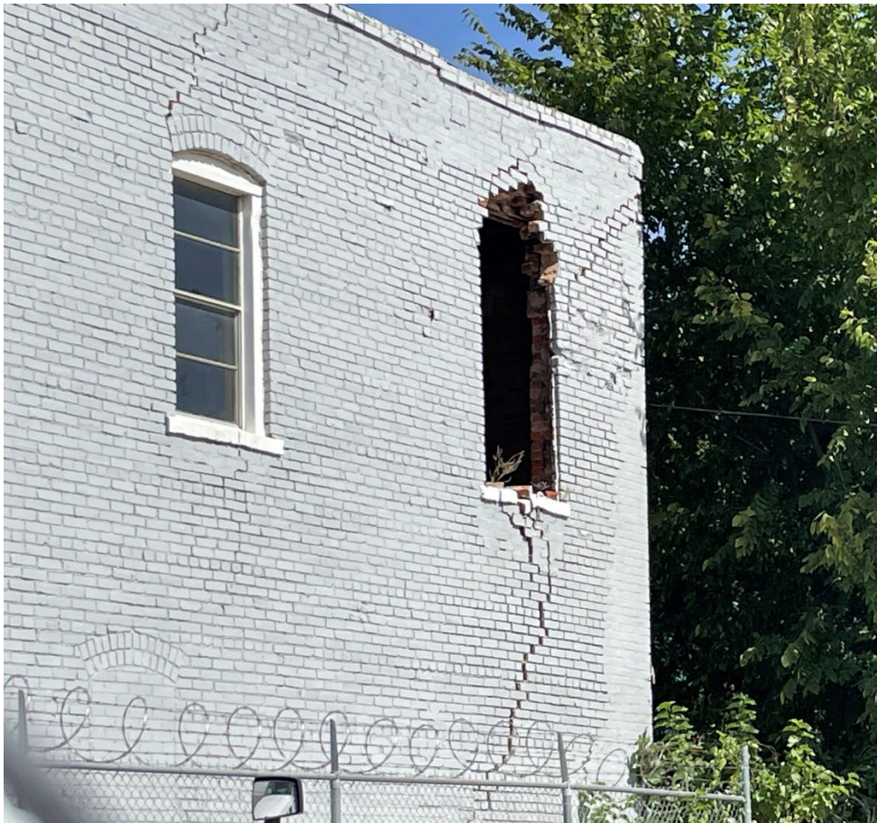
Figure 27. Site photos July 3, 2024, missing window and deteriorated wall.
