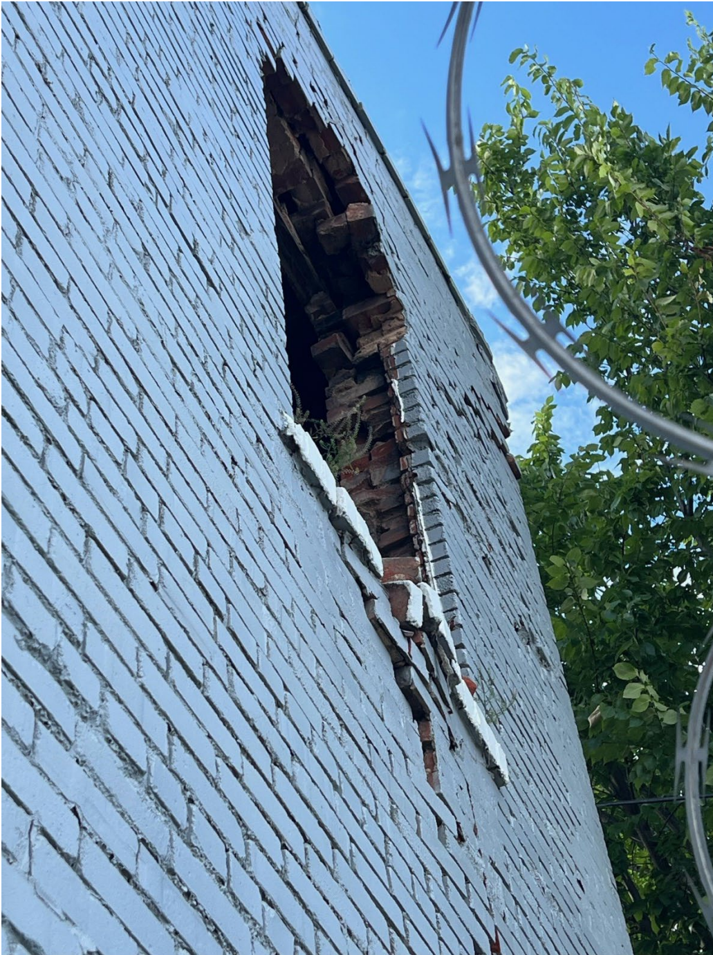
Figure 17. Picture of the failing wall June 13, 2024.
