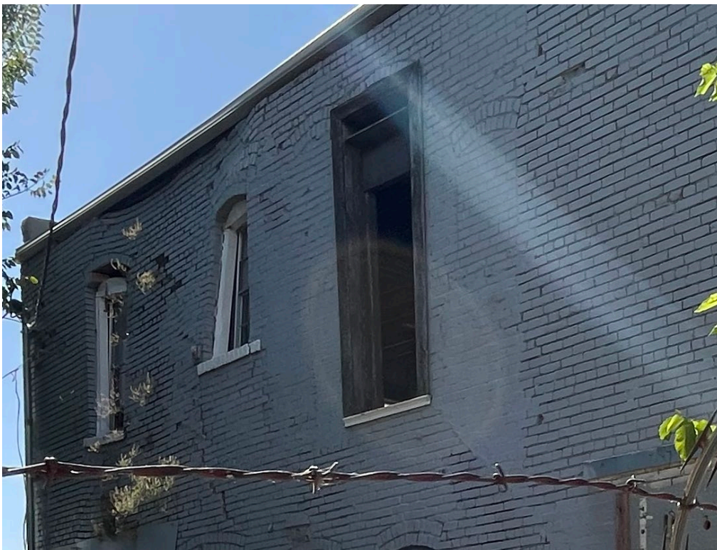
Figure 25. Site photos July 3, 2024, deteriorated windows.
