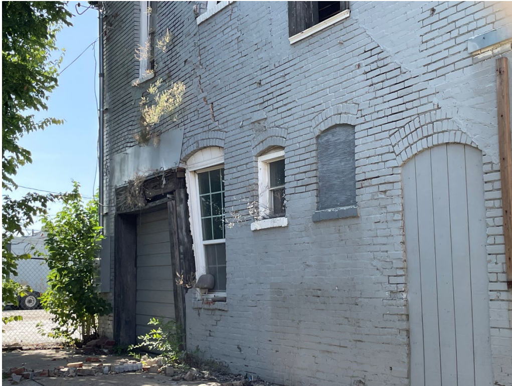
Figure 24. Site photos July 3, 2024, deteriorated window, overhead door, enclosed window.
