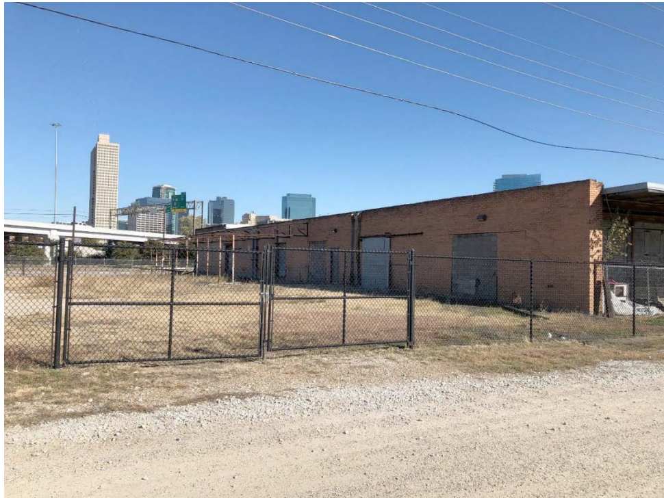
Fig. 6 – Western elevation. The west elevation of the original building is fully obscured by the addition shown here.
