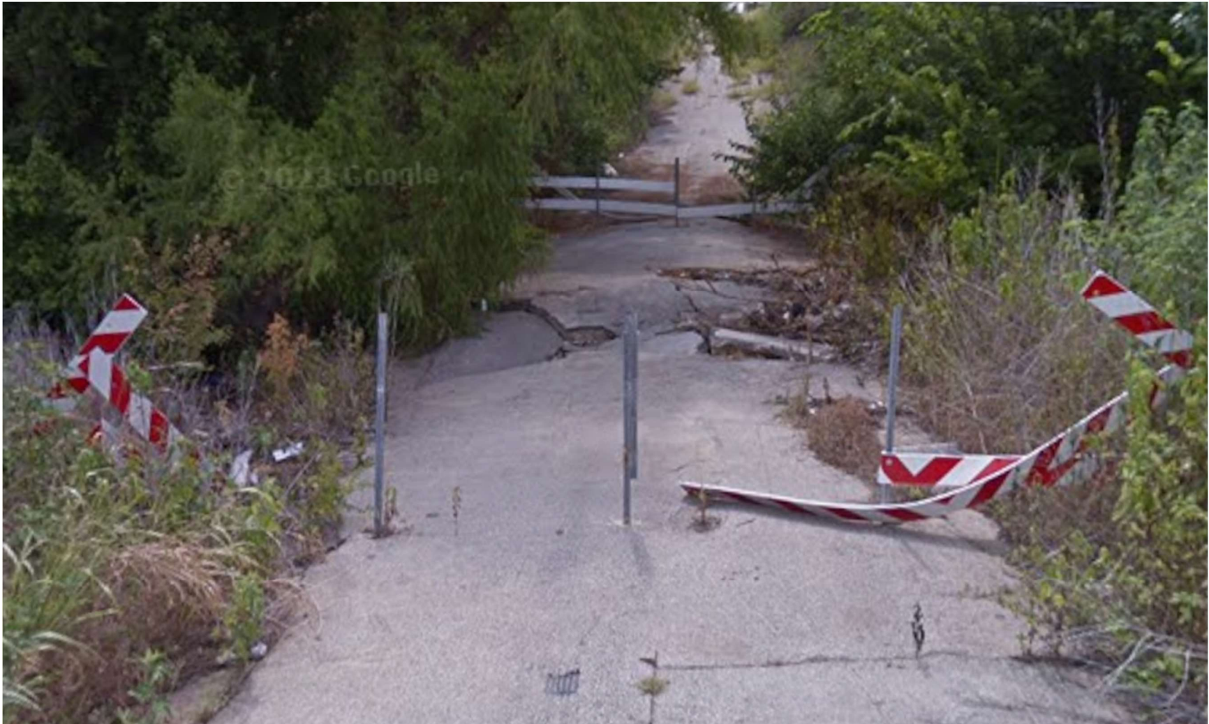
Farnsworth Avenue Roadway Washout, Face View Current Conditions, Looking East
