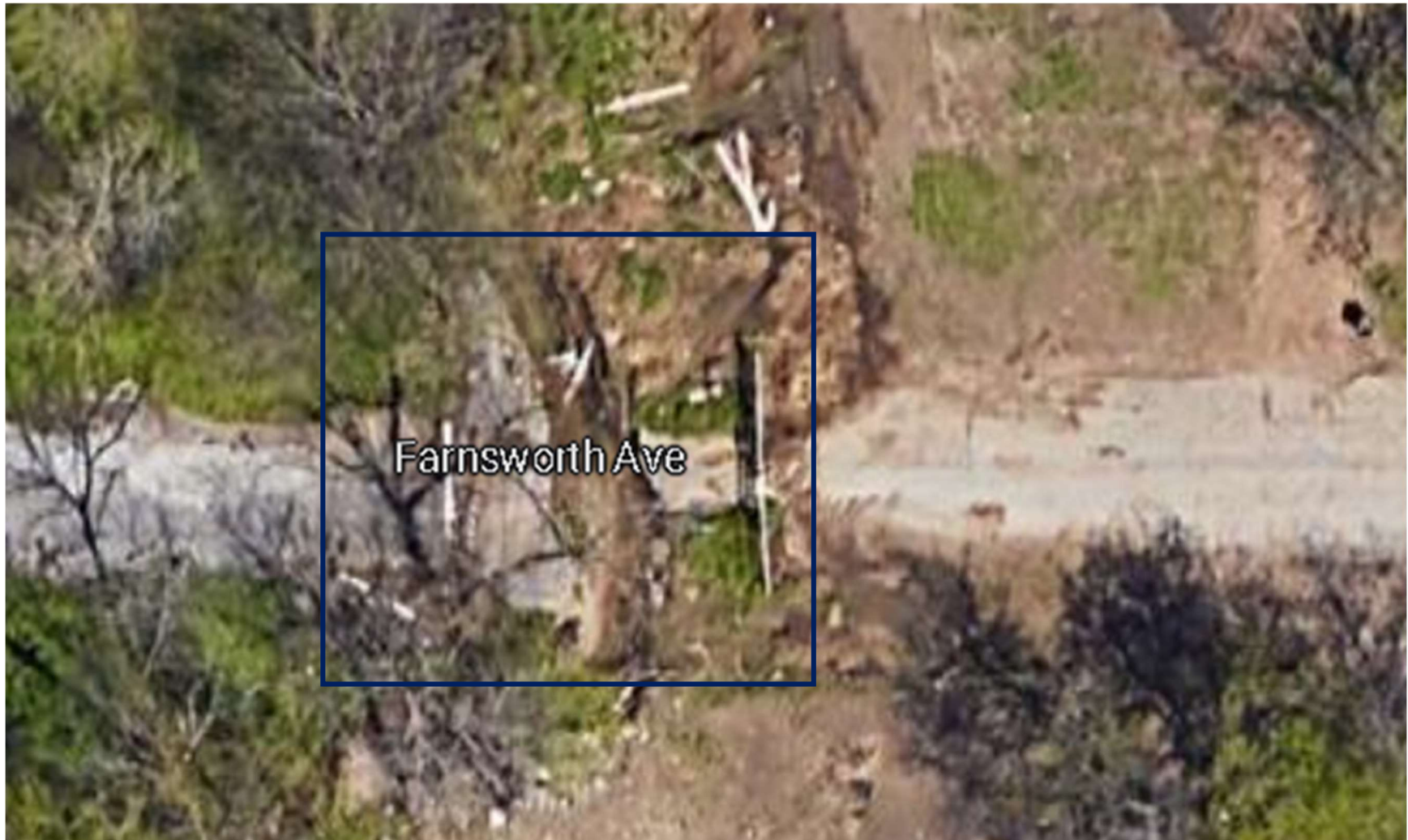
Farnsworth Avenue Roadway Washout, Aerial View Current Conditions
