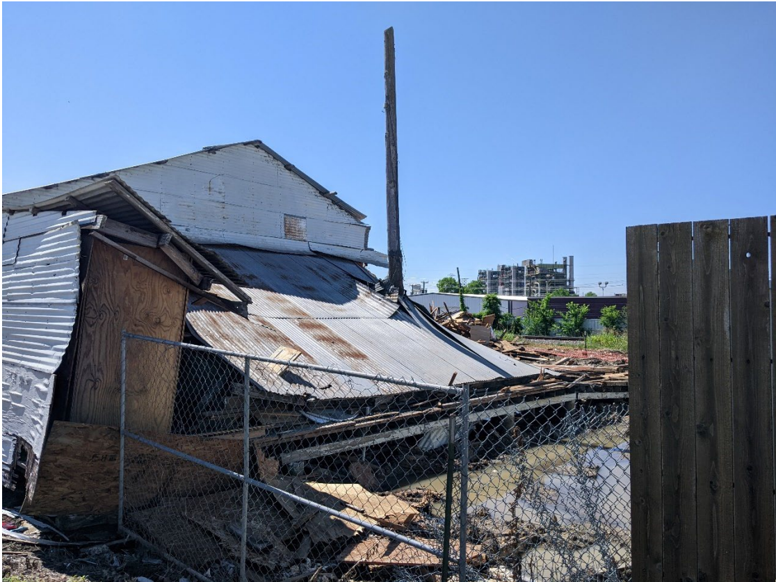
Figure 5. Subject property May 2024 after Stop Work of illegal demo was issued.
