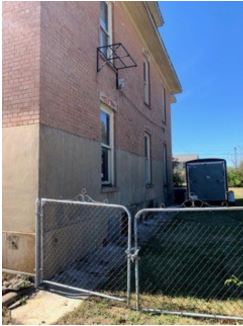
Fig. 8 – Right elevation. Note masonry cladding, which is very similar to construction methods used in the Stockyards on in industrial architecture, where Mr. Koldin worked.
